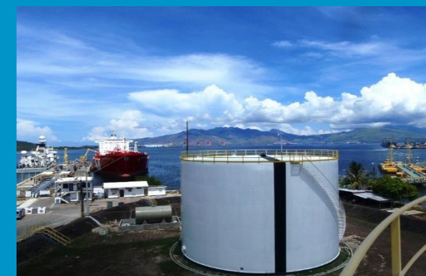
Petroleum and petroleum products pipeline transmission or distribution systems
