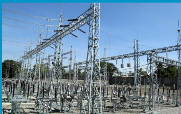
Distribution of Electricity
